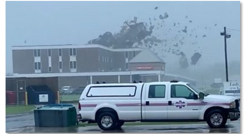
Lady of the Sea Hospital, Galliano, Louisiana Hurricane Ida, 2021
